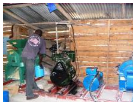
MFP plant installed at Leguruki
