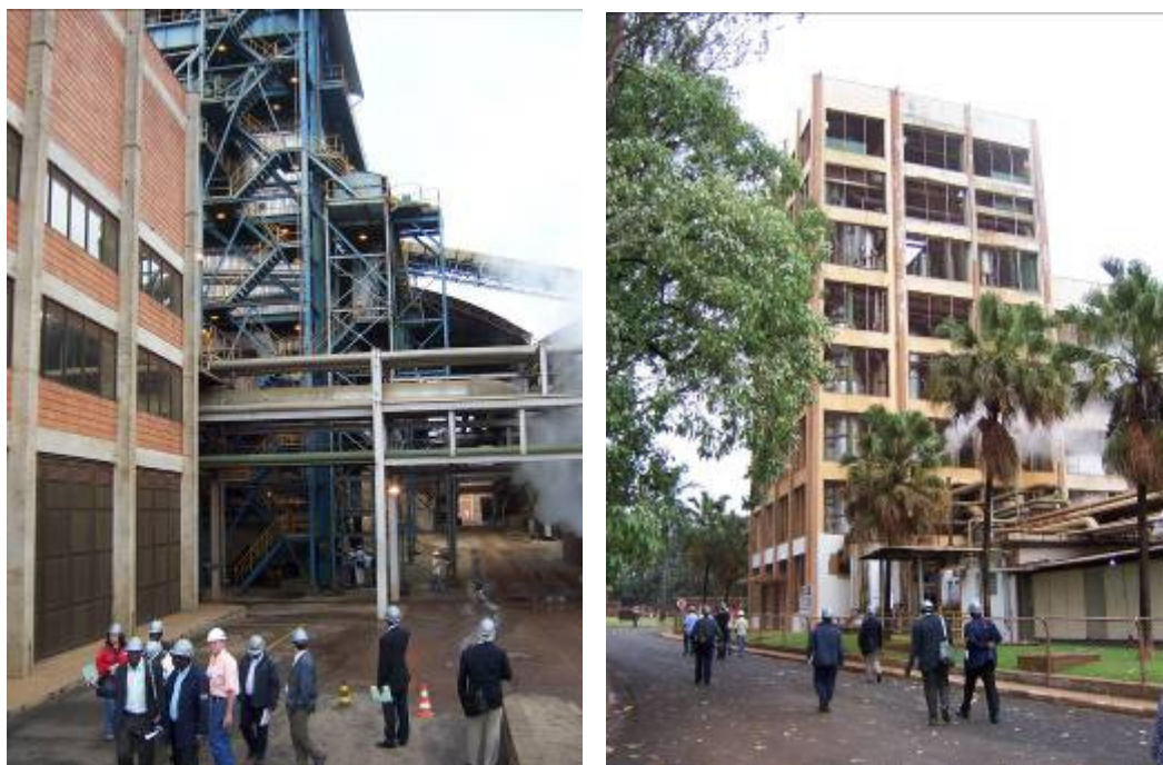
High pressure boiler (left) and bioethanol distillery (right) at Santo Antonio Sugar Factory, Brazil
